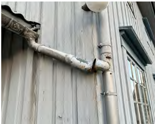
Figur 90 – Brudd i takrenner.
